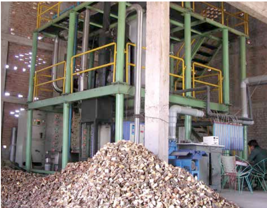
▼ A view of a gasifier plant and fuel from Bihar...
